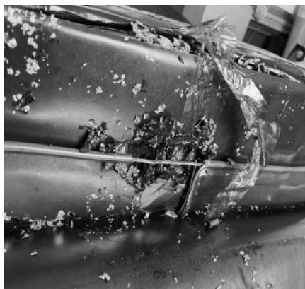
图9 故障电容单元解体图 Fig. 9 Disassembly diagram of faulty capacitor unit
